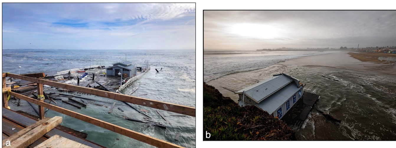
Figure 26. (a) Outer end of the Santa Cruz pier after collapsing into the ocean on 23 December 2024 (photo credit: Brad Porter, City of Santa Cruz). (b) Restroom from end of municipal wharf was carried intact where it floundered on the beach at the mouth of the San Lorenzo River (courtesy of: Kevin Painchaud, Lookout Santa Cruz).
