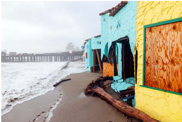
Figure 22. Late December 2023 storms further damaged the beach-level Venetian Court (photo credit: Kevin Painchaud, Lookout Santa Cruz).
